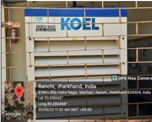
Generator: Capacity 82.5 KVA(Krilosker)
