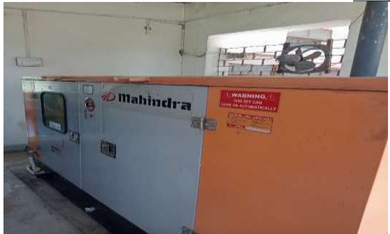
Generator: Capacity 40KVA (Mahindra)
