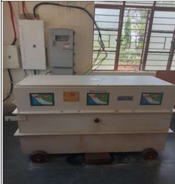
Stabilizer : Capacity 63 KVA
