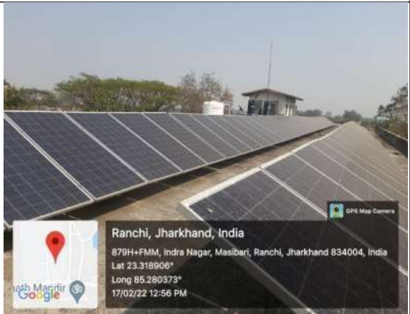
Solar Panel 99 plates : Capacity 30 KW
