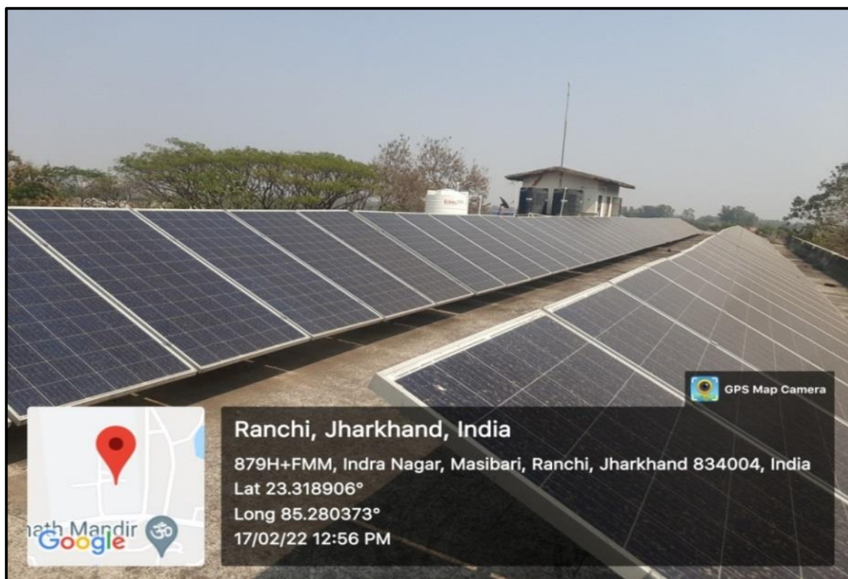
Rooftop Solar Panels-Geotagged photograph of the facility,
