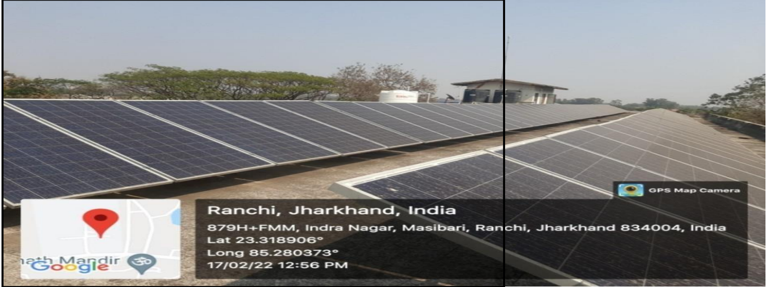
Rooftop Solar Panels-Geotagged photograph of the facility (2019)
